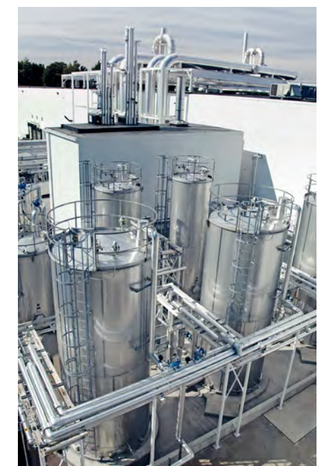
Solvent distillation column and tank farm
